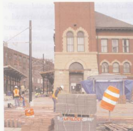
The Broad Street Station project combines significant upgrades to bring the building up to modern standards and extensive restoration or duplication of historic elements.
